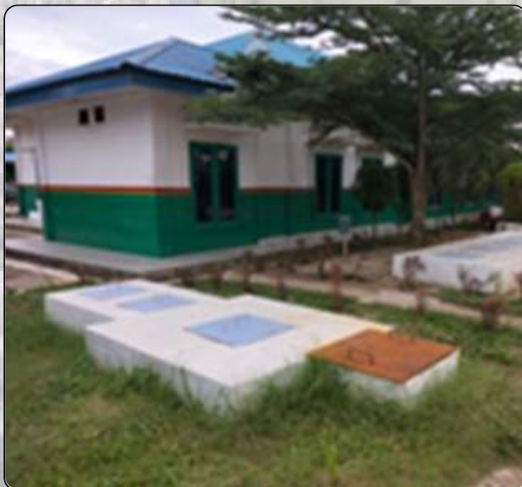
Domestic Wastewater Treatment Facilities in PT SUAN IPAL Domestik di PT SUAN
